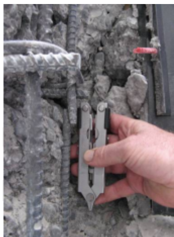
Figure 6: Fractured bars in lightly reinforced wall
