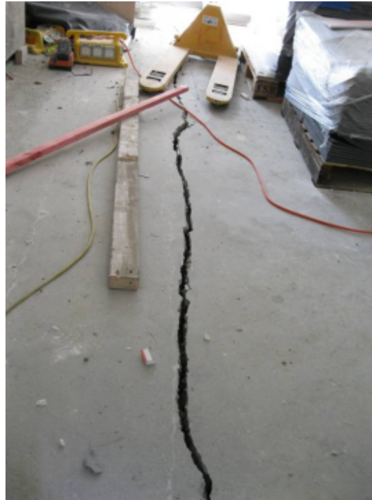
Figure 9: Floor tearing caused by frame elongation
